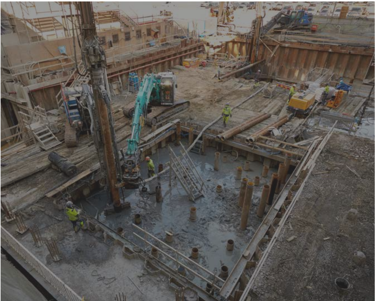
Image above: Nordisk Bergteknik's subsidiary Pålab performs piling work for the now completed Hotel Draken at Järntorget in Gothenburg.
