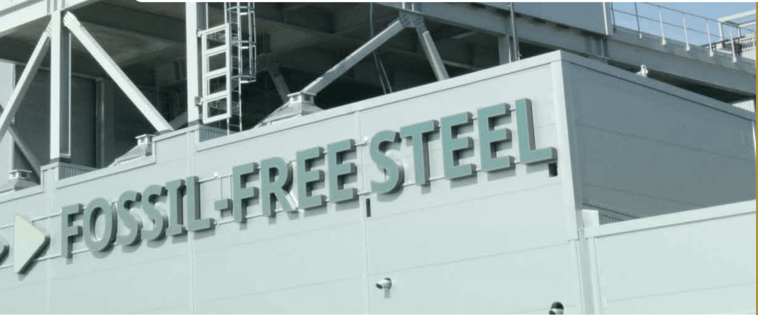
Nordisk Bergteknik's subsidiary Norrbottens Bergteknik during the construction of the rock shelter storage for fossil-free hydrogen in Luleå
